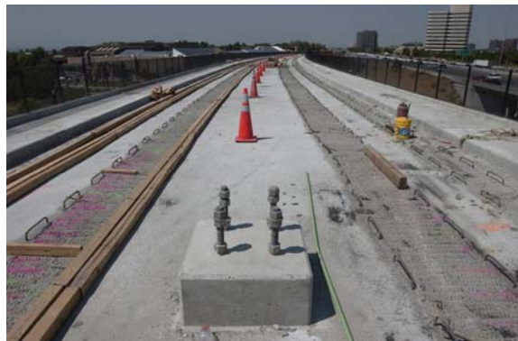
Figure 7. Concrete plinth construction. Note the exposed “crank-shaft” shaped bars at the plinth and deck interface locations.
