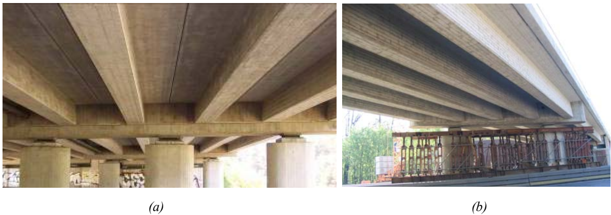
FIGURE 3 Precast, Prestressed Bridge on Autobahn near Munich, Germany: (a) T-Beams with Integral Bent Caps; (b) Temporary Shores for Beams.
