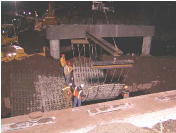
Figure 10. Precast block scour blankets
