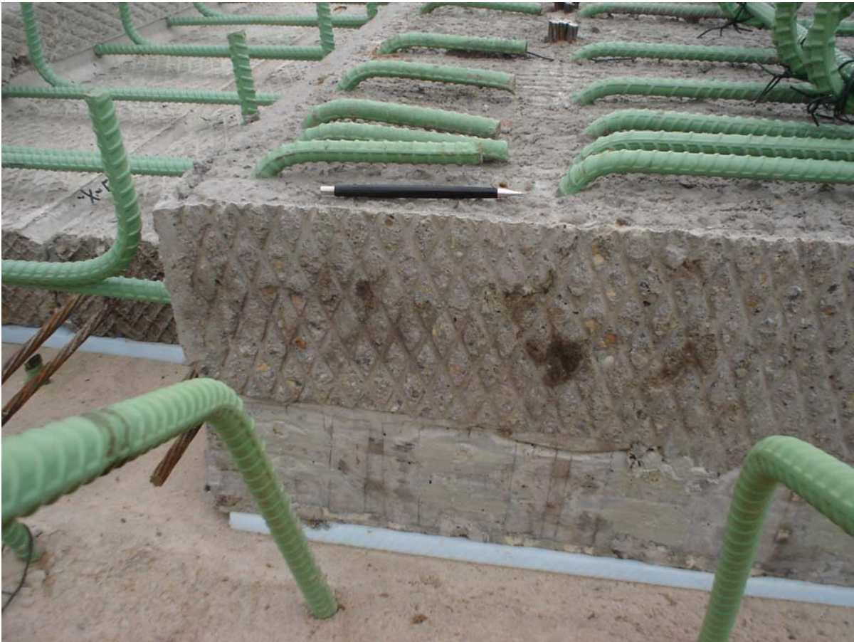
Figure 9. Final Roughened Surface. The surface shown on the side of the beam is typical for all formed contact surfaces except for the top of the beam. The top of the beam is broomed transversely.
