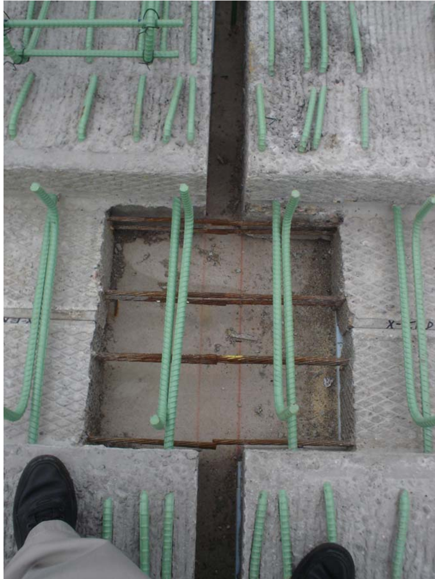
Figure 7. Pier Blockout Detail at Construction – Center City Bridge. In this photo the pier is running vertically and the beams are running horizontally. Anchor rods still need to be drilled into the pier cap.
