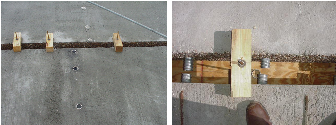
Fig. 11 Wood forming of the panel-to-panel joint used in the Arch Tied Bridges, Texas
