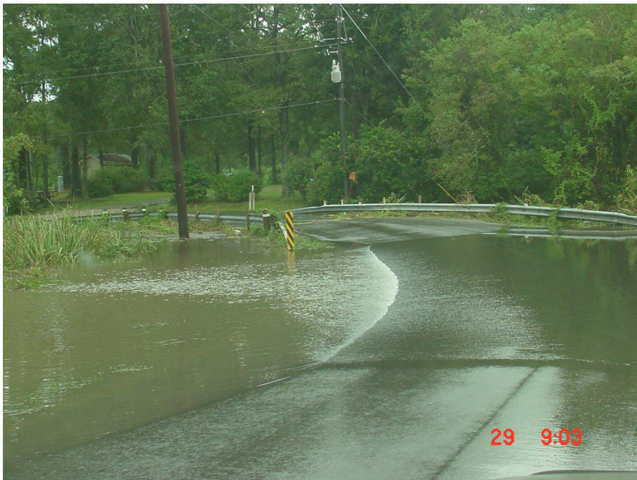
Fig. 3 Existing Structure During Heavy Rainfall.
