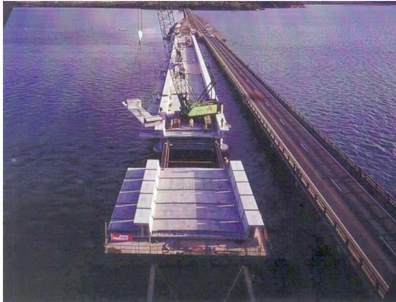
Figure 10. Installation of Channel Segments of Sorell Causeway Bridge (source: Gibbens and Smith 2003)
