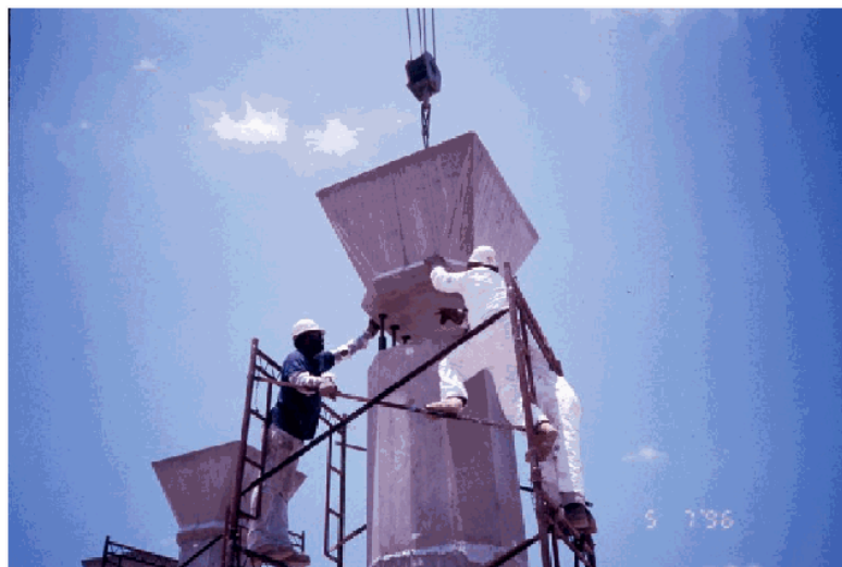
Figure 15. SH 249/Louetta Road Overpass (Source: www.aashtotig.org , Photo Credits: Texas Department of Transportation)
