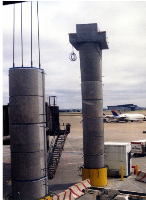
Figure 14. Dallas/Fort Worth International Airport People Mover (Source www.aashtotig.org , Photo Credits: STOA/Carlos + Law, AE)
