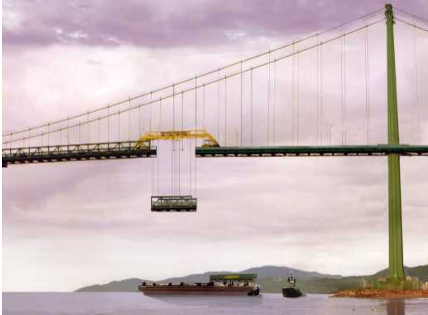
Figure 12. Lions' Gate Suspension Bridge (source: www.aashtotig.org . Photo credit : British Columbia Ministry of Transportation)
