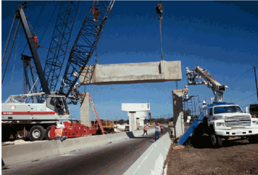
Fig. 13. US 290 Ramp E-3 Bridge (source: www.aashtotig.org Photo Credits: Texas Department of Transportation)
