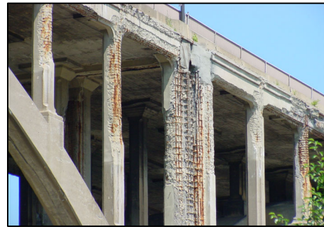
Deterioration of Existing Structure
