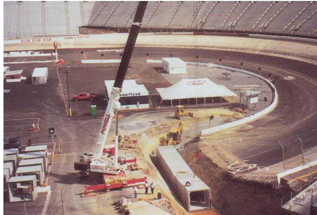
Fig. 7 NASCAR Race Track Service Tunnel, Bristol, Tennessee 2001
