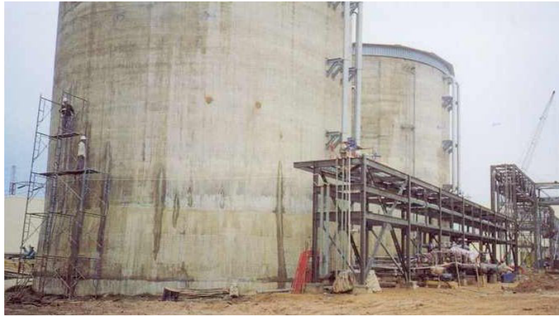
Fig. 19 Electricity Power Plant, Vietnam, 2001
