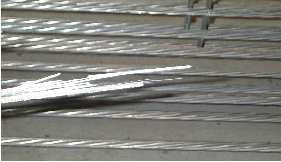
Fig. 5 CFRP wire rupture due to shock wave after initial slip
