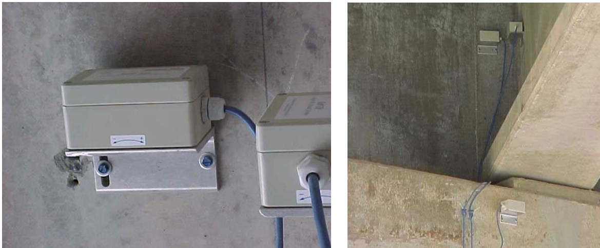
Fig. 11 Typical tiltmeter installation
