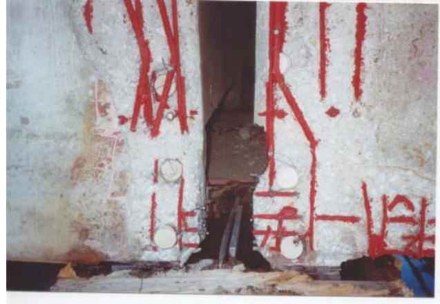
Photo 4 Prestressed beam end with galvanic anodes and rebar coating installed prior to concrete replacement.
