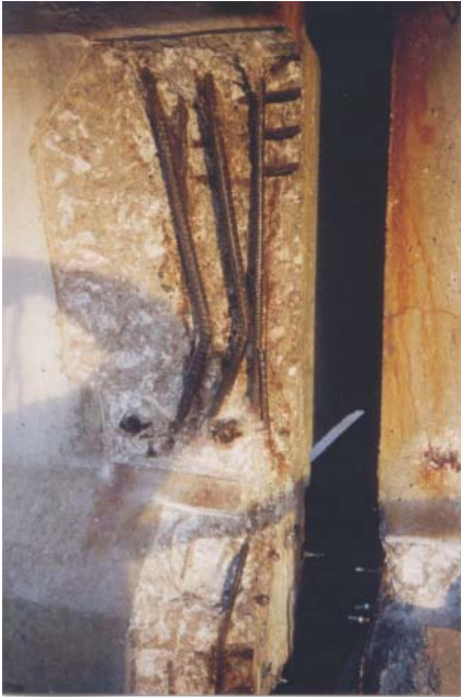
Photo 3 Prestressed beam end subject to corrosion
