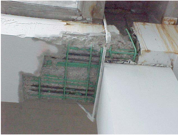
Photo 2 Precast/prestressed beam repair. Delaminated concrete cover removed but strands remain partially embedded in chloride-contaminated concrete.
