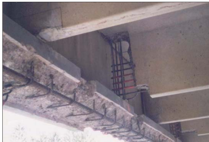
Photo 1 Precast/prestressed double T beams ends suffering from chloride-induced corrosion.
