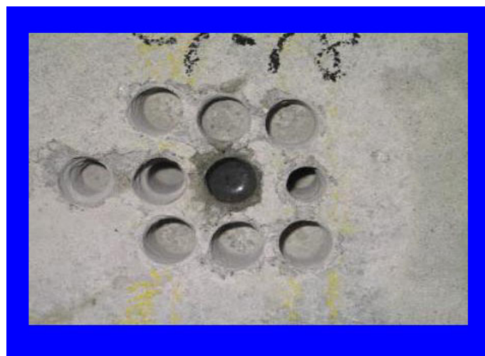
Fig. 13: Water seeping from drilled hole
