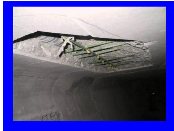
Fig. 15: Water entering ungrouted temporary tendons, creating freeze-thaw damage inside the top slab of segment
