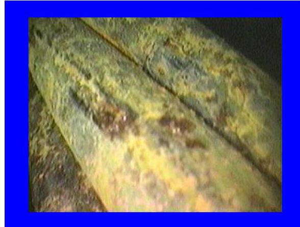
Fig. 14: Slight onset of strand corrosion
