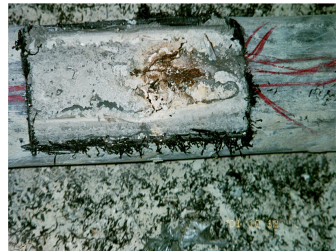
Fig. 7 Localized Strand Corrosion at Hole
