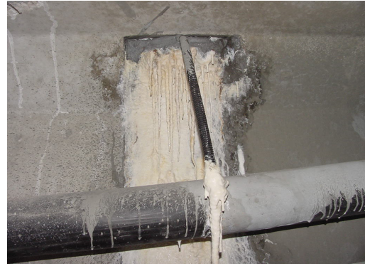
Fig. 14 Efflorescence from Anchorage
