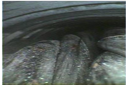
Fig. 11 Void in Top of Duct Recent Construction
