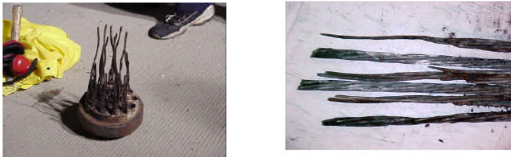
Fig. 18 Condition of Removed Tendon at Anchorage
