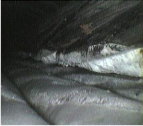
Fig. 8 Void With Strands Exposed
