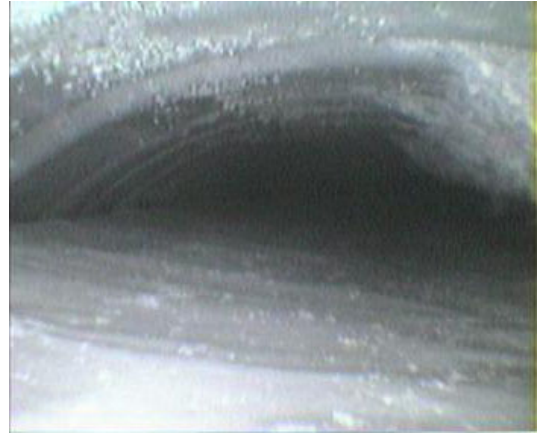
Fig. 9 Void without strands exposed
