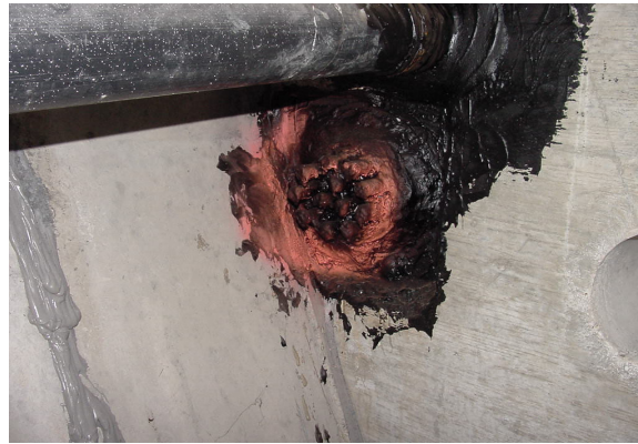
Fig. 15 Exposed Unprotected Anchorage
