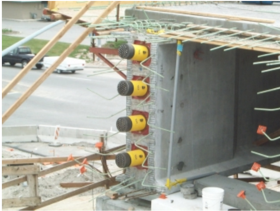
Fig. 5. Load Cells 1 thru 4 on the North End of Girder A after post-tensioning
