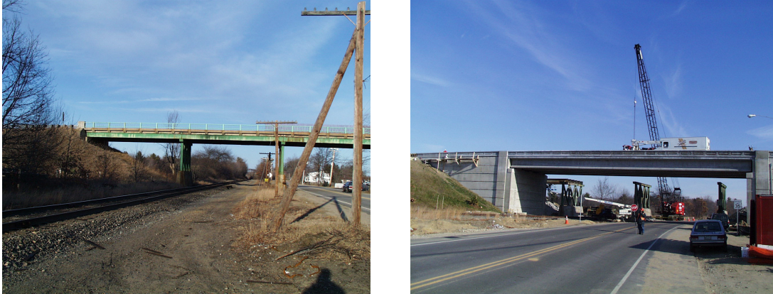
Figure 1: Before (left) and after construction (right) photos of the Rollins Road Bridge.
