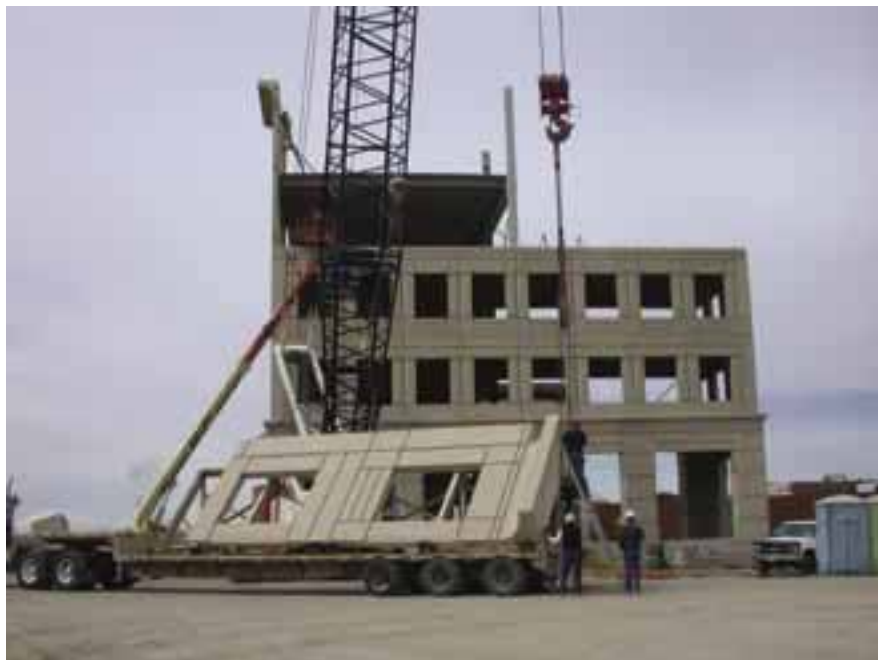
Fig. 17. Weighing 34,000 lb (15,422 kg), a 32 x 10 ft (9.8 x 3.1 m) loadbearing precast concrete wall panel is tripped from the flatbed.
