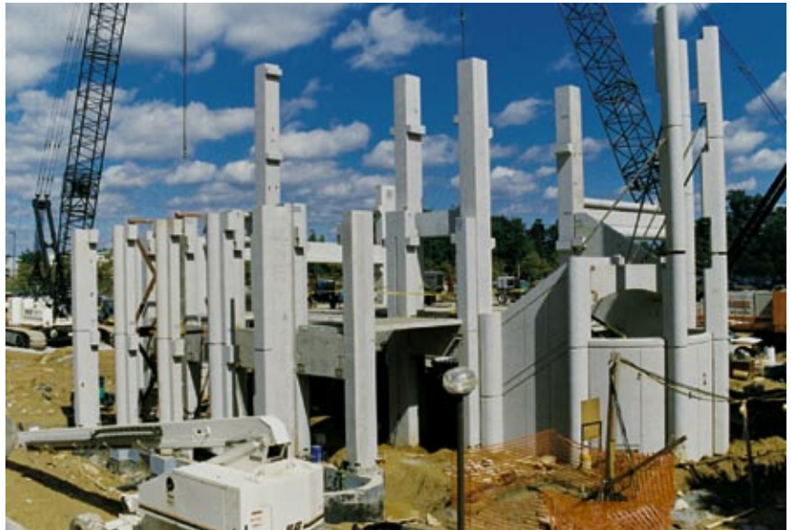
The total-precast design includes shear walls, inverted tee beams, spandrel beams and double tees. Here, columns for one of the stair and elevator columns are erected. Photo: ©FineArtPhotography.com
