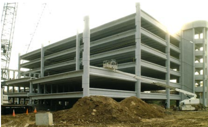
Major exterior columns were rounded on the exterior face to maintain the rounded theme used throughout the project. Photo: ©FineArtPhotography.com
