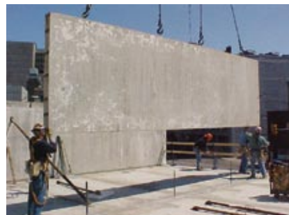
Each 28-foot section of precast concrete wall panel was set and anchored in about one hour.
