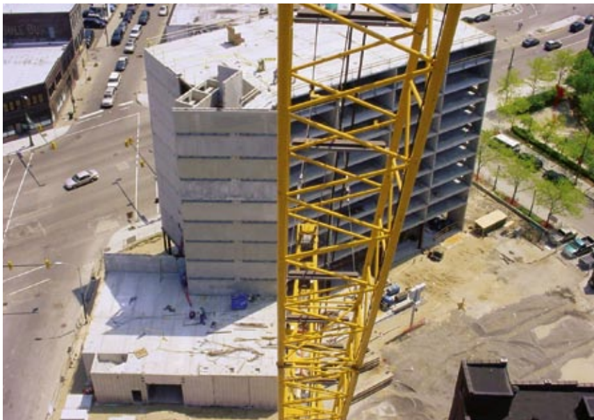
The site offered tight restraints, requiring the team to rent the adjacent parking lot to provide space for the crane during the erection process.
