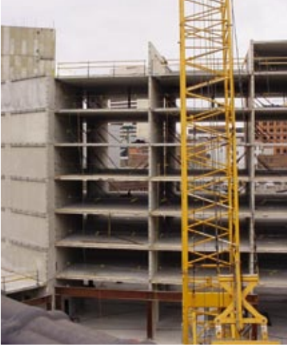
Construction crews coordinated with the precaster to saw-cut openings as needed on each level.
