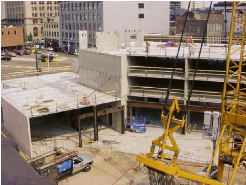
The hotel features a modified L shape and was constructed in two phases to allow interior crews to begin finishing one section quickly.
