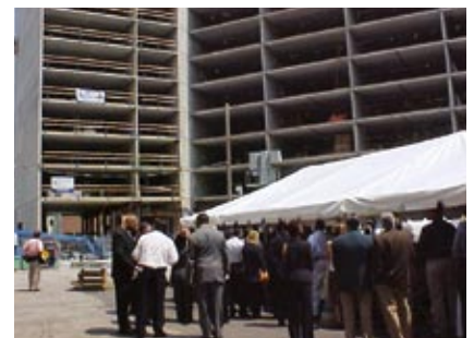
Eight-foot-wide hollowcore planks were used as flooring on each level to reduce joints and picks.
