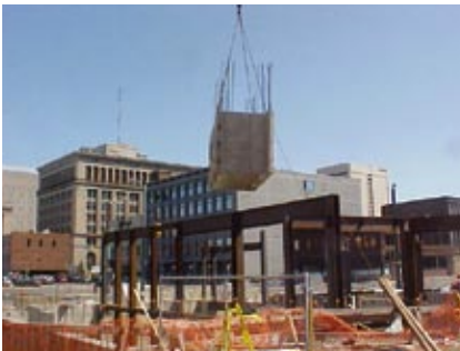
A 260-ton-capacity crane lifted the 52,000-pound precast "boxes" used for elevator shafts.
