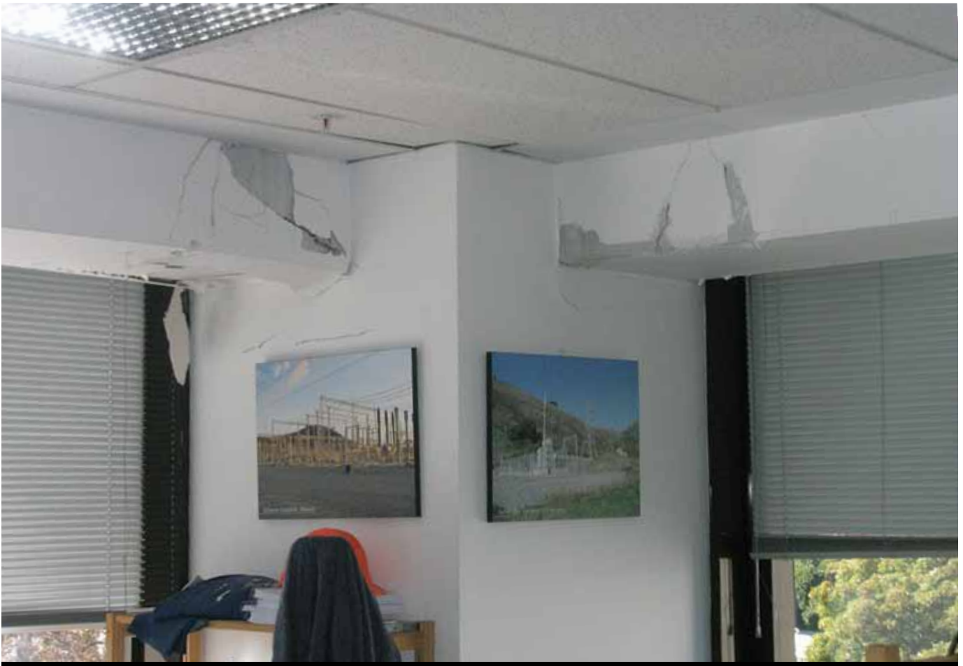
Figure 4. Corner joint in upper floor indicated damage suffered in February 22, 2011, earthquake in New Zealand. The north-south beam (upper left) exhibits flexural-torsional cracks, while the east-west beam (upper right) exhibits flexure cracks.
