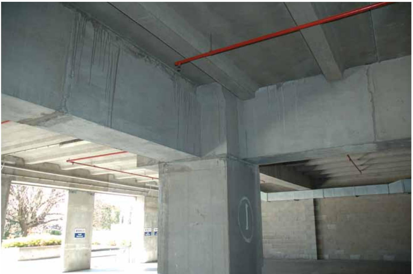
Figure 3. Corner joint in first-level parking podium area after February 22, 2011, earthquake in New Zealand. Photo courtesy of Franz Kahn.
